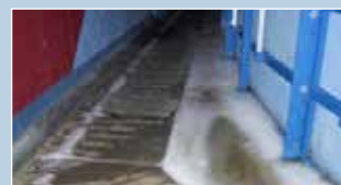
BEFORE Uninsulated brine headers are causing frosting and unsafe conditions as well as not being energy efficient.
